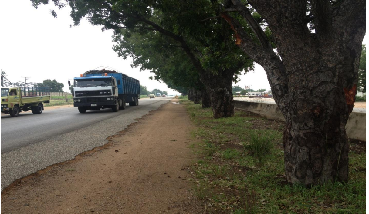
Picture 4 (P4) Dangerous trees on the road median km 38+700
