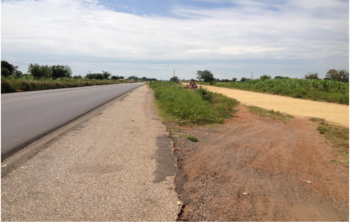
Picture 6 (P6) Improper placements of vertical sign km 23+200
