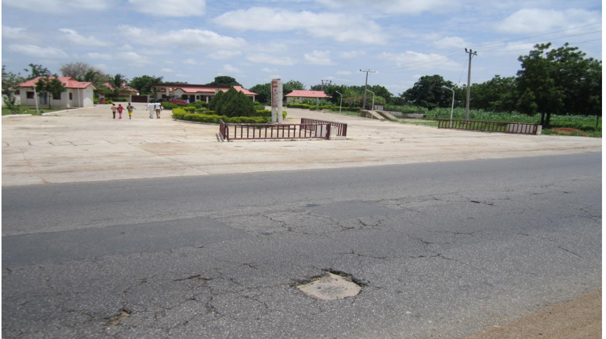
Picture 7 (P7) Improper connection to petrol station km 21+500
