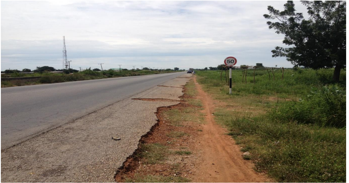
Picture 22 (P22) Speed limit too low km 28+600
