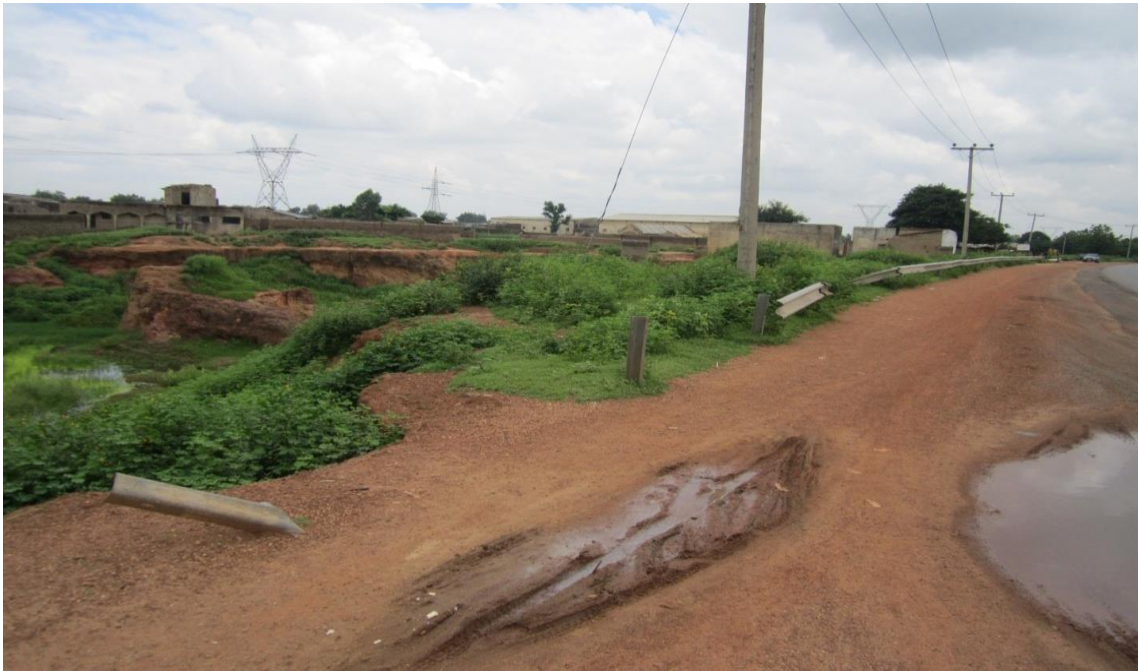
Figure 4.10 Dangerous Guardrail Section (Km 21+500)
