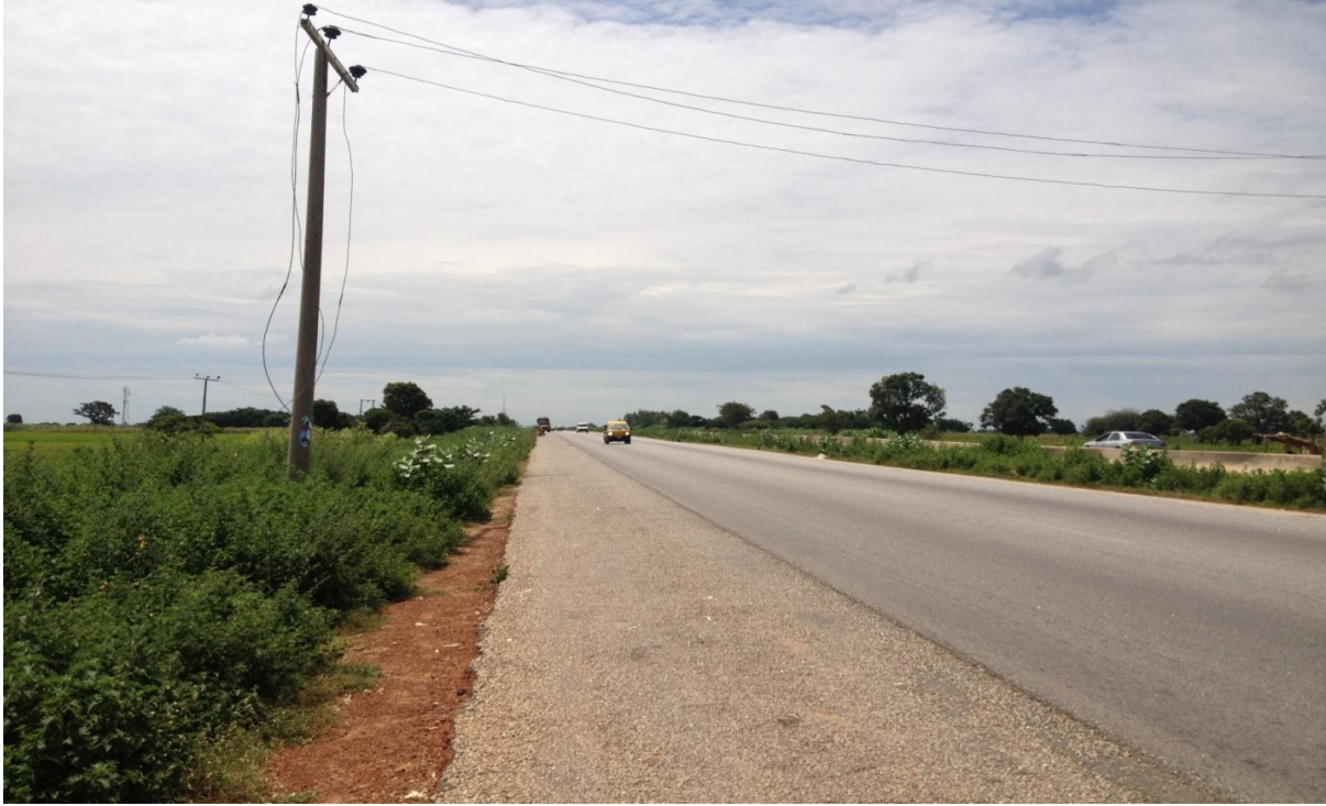
Picture 2 (P2) Dangerous electric poles close to the roadway km 47+200
