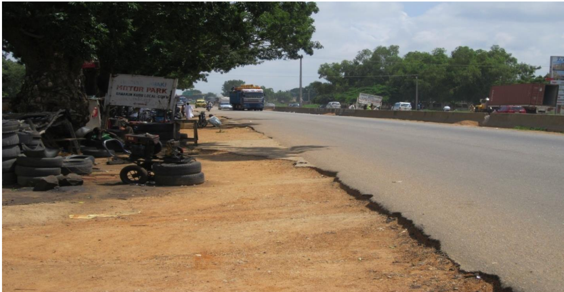
Figure 4.13 Dangerous Tress, Signboard And Objects Close to the Roadway (Km 3+200)
