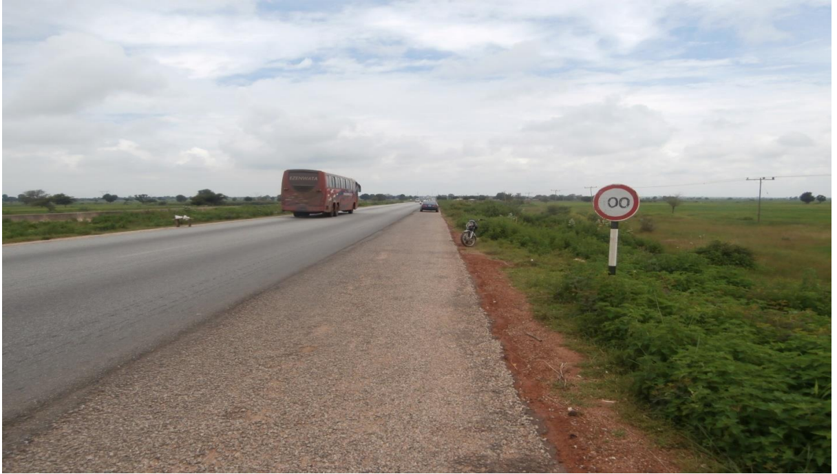
Picture 5 (P5) Warn out vertical sign km 10+700
