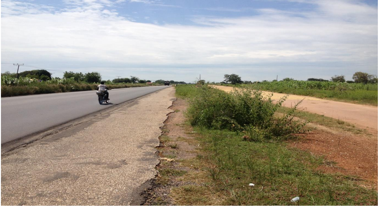
Picture 20 (P20) Improper placement vertical sign km 30+500
