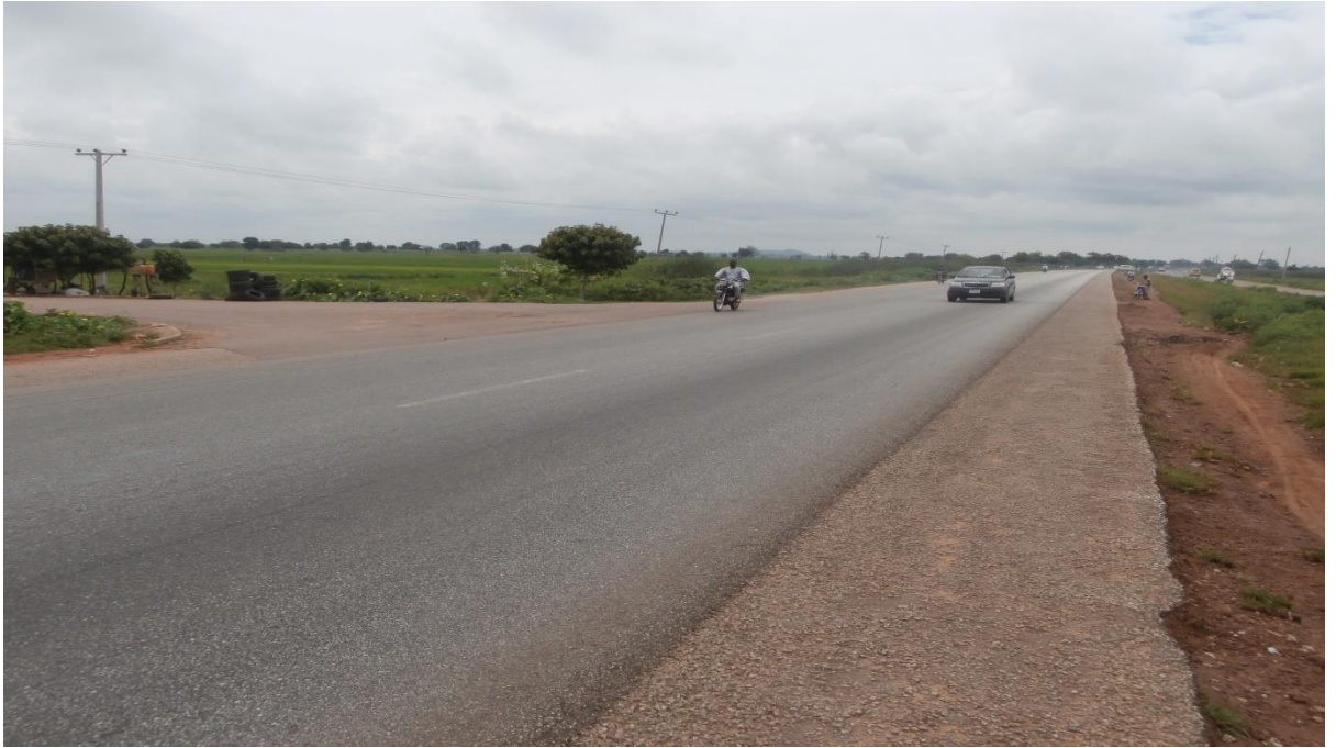
Picture 24 (P24) Improper junction design km 24+900
