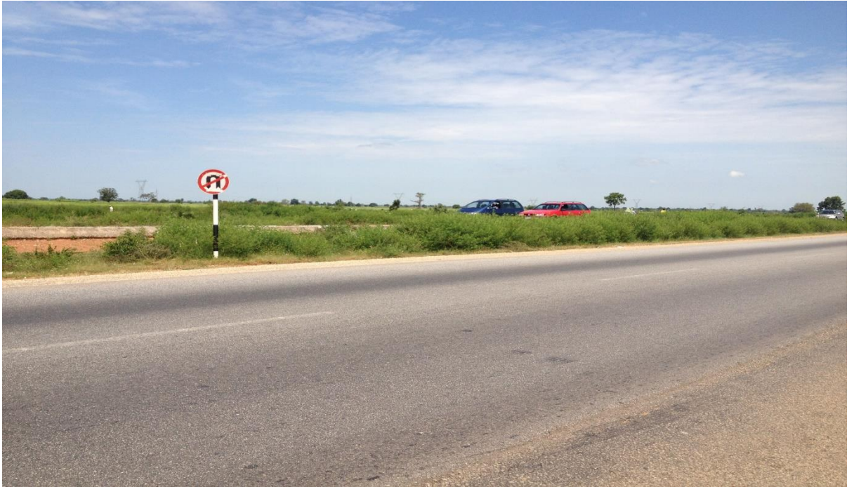
Picture 21 (P21) Confused warning sign km 41+700
