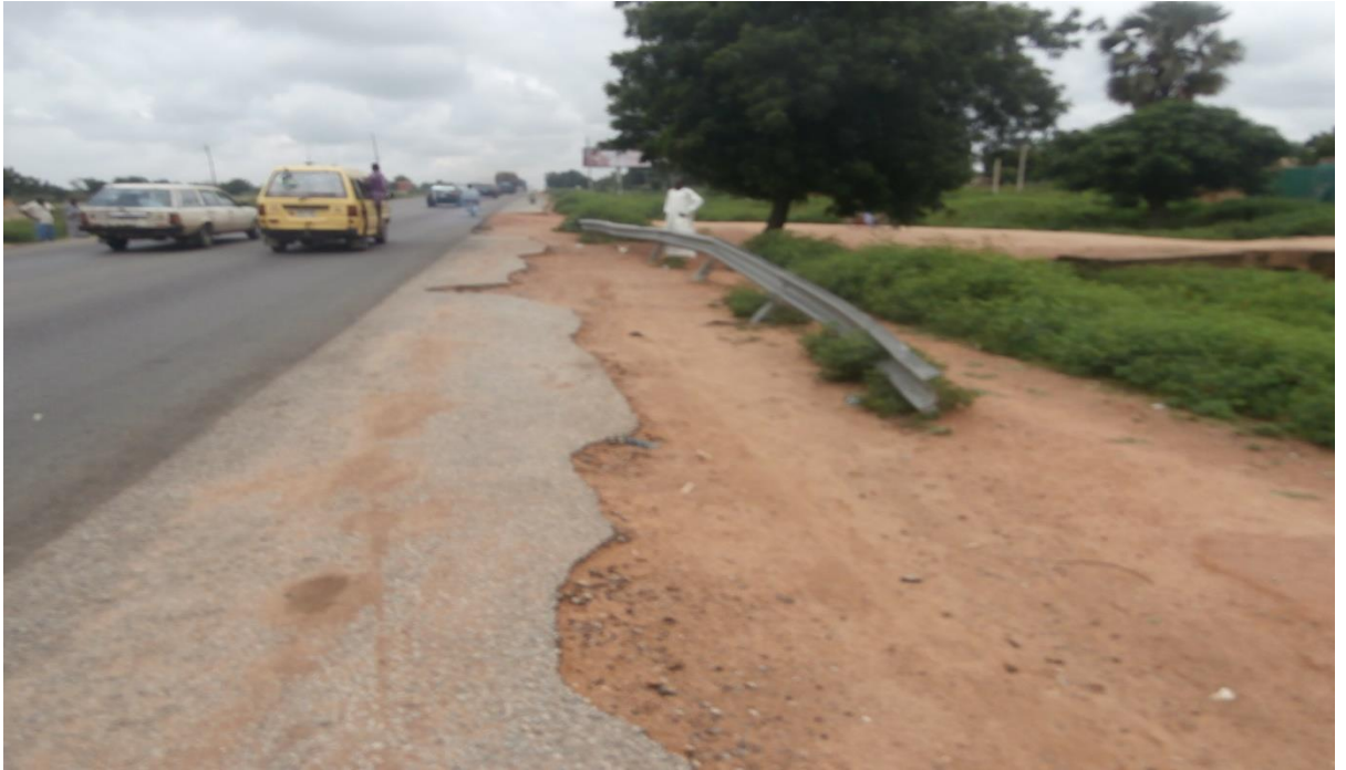
Picture 19 (P19) Dangerous guardrail start km 49+100
