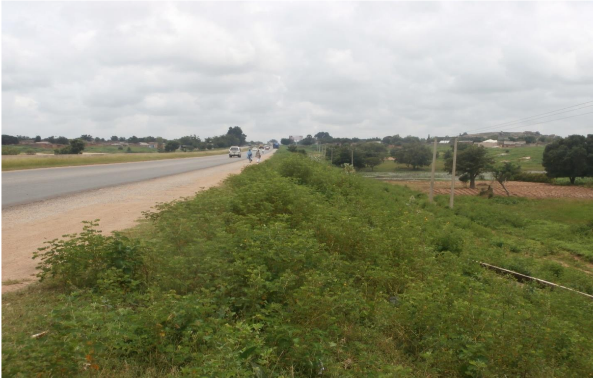
Picture 10 (P10) Dangerous fill slope km 4+400
