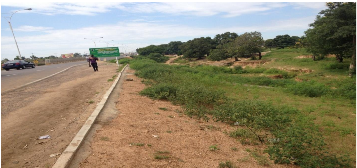
Figure 4.9 Dangerous Fill Slope (Km 2+700)
