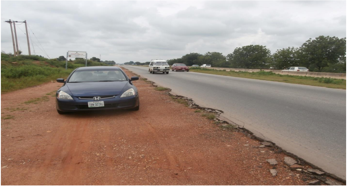
Picture 9 (P9) Missing shoulder and edge deterioration km 40+100
