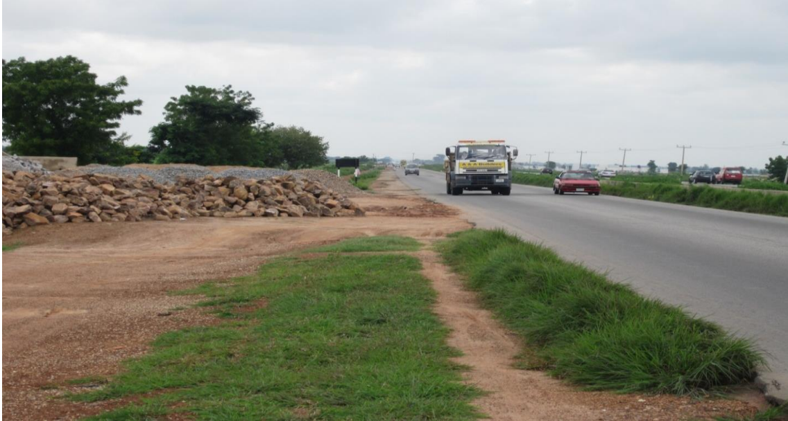
Figure 4.8 Shoulder Missing (Km 44+100)
