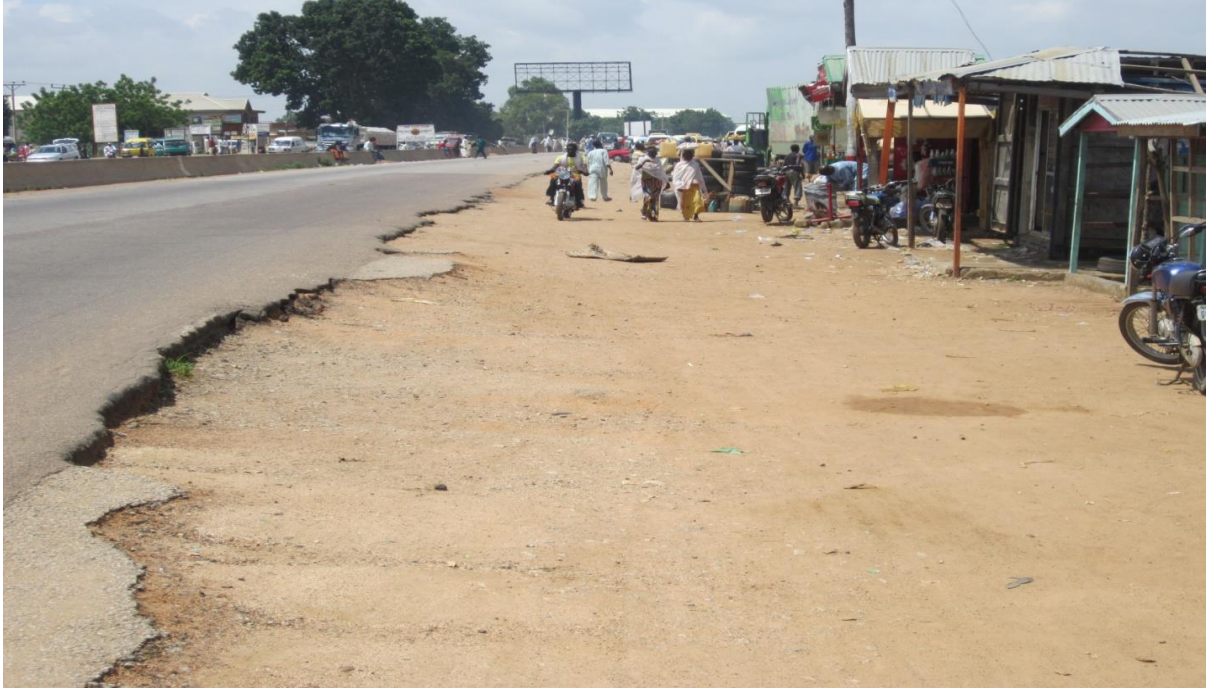
Picture 17 (P17) Missing safety zone km 15+600
