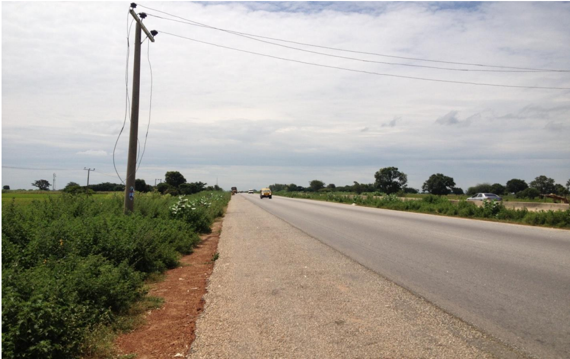
Figure 4.3 Dangerous Electric Poles Close To the Road (Km 47+200)
