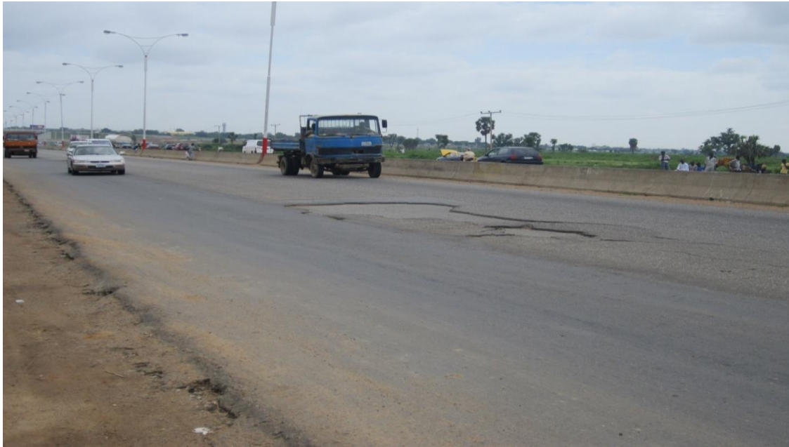
Figure 4.11 Dangerous Potholes on the Pavement (Km 9+00)
