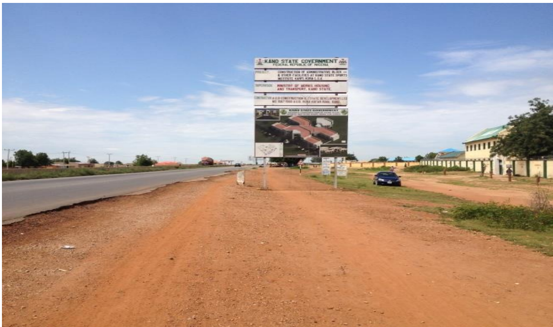
Figure 4.12 Improper Placements of Vertical Sign within the Safety Zone (Km 6+400)
