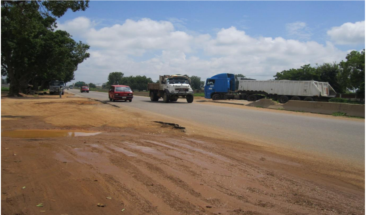
Picture 18 (P18) Improper median opening km 23+300
