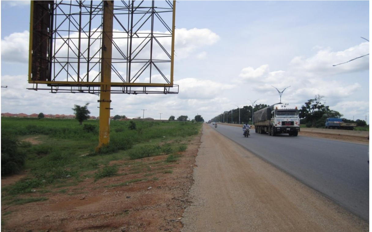
Picture 12 (P12) Dangerous support for advertisement km 32+700
