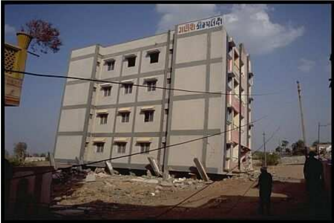
Figure 1.1. A building that has been collapsed in an earthquake as a result of soft story behaviour.
