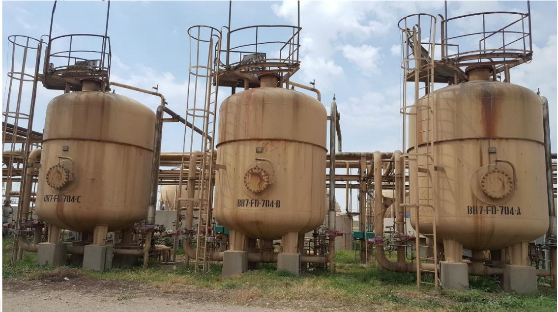
Figure 1.3 Sand filters A, B, C
