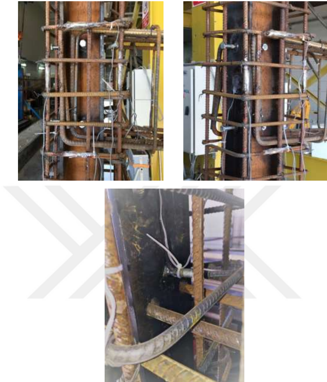
Figure 3.13 Congested beam steel hooks inside the joint
