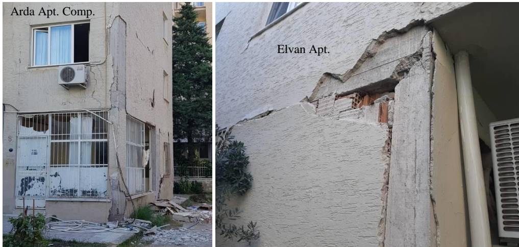
Figure 30. Severe column damage
