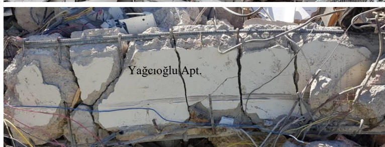
6 Figure 36. Reinforcement configurations of the columns and beams of the collapsed buildings
