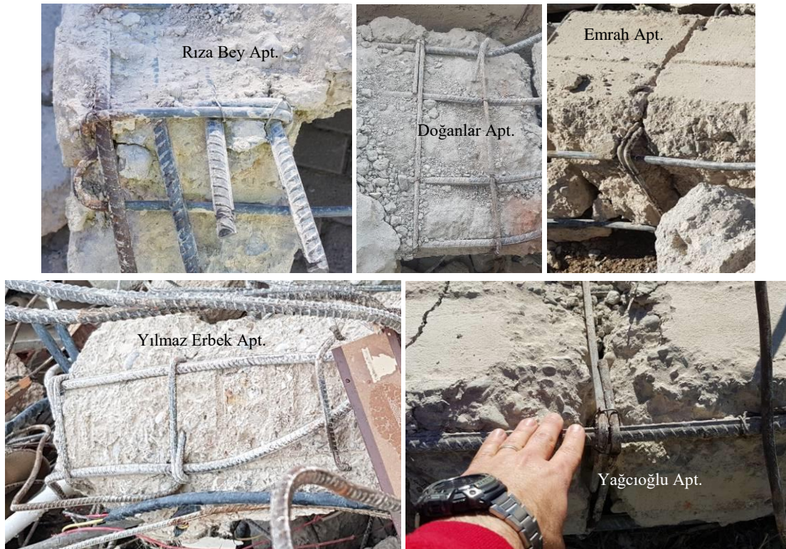
Figure 37. Ends of the stirrups (bent 90°) of the collapsed buildings
