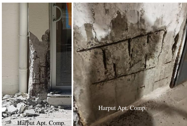
11 12 Figure 35. Corrosion of reinforcements due to moisture
