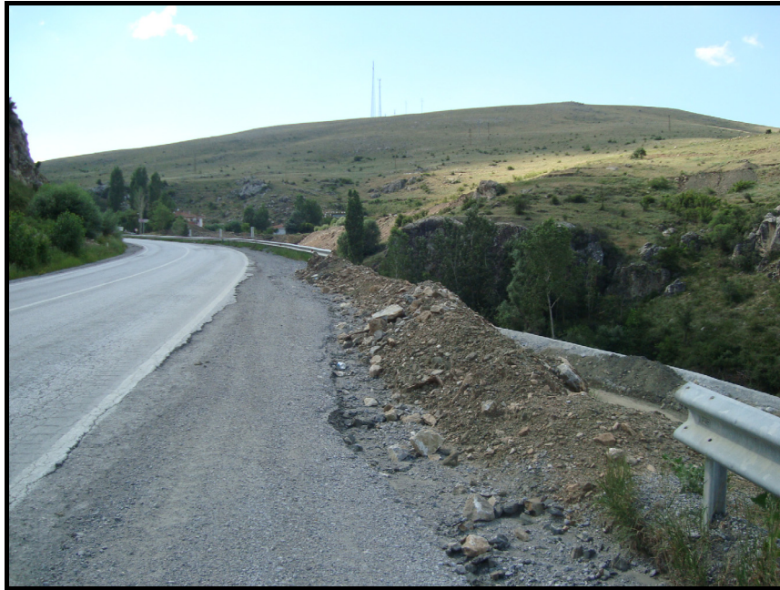
Figure 4.16 Dangerous guardrail section
