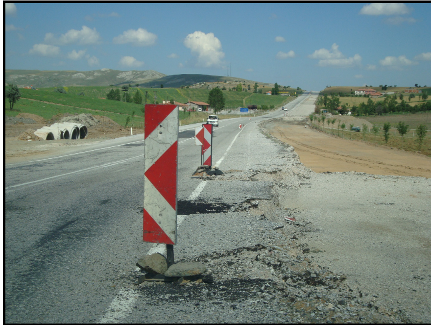
Figure 4.18 Improper location of warning sign
