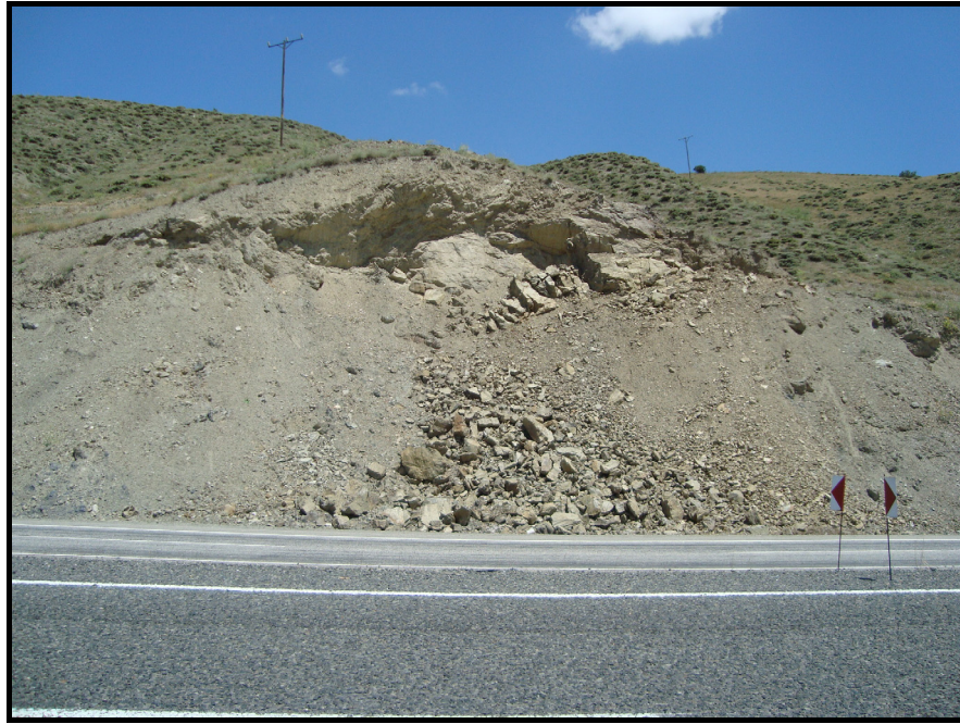
Figure 4.15 Dangerous cut slope area
