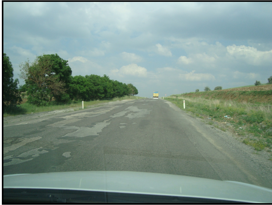
Figure 4.17 Improper pavement design
