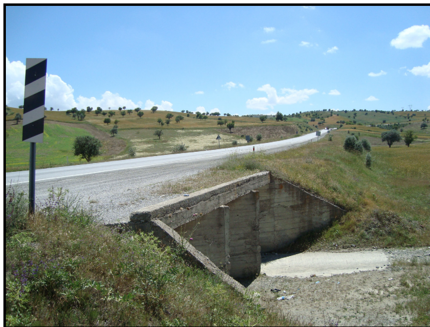
Figure 4.10 Dangerous transition zone of culvert without guardrail
