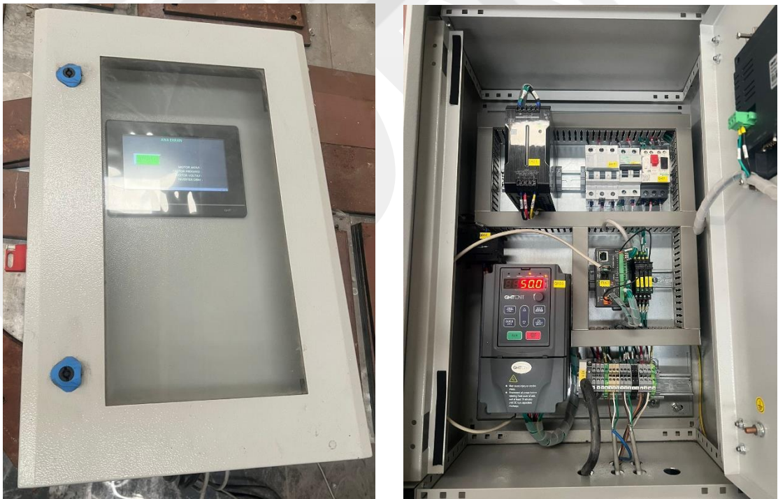
Figure 4.5: Control panel outside and inside view.
