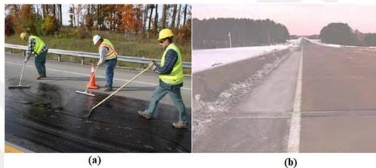
Figure 1.3 (a) The application of PC with epoxy as a cover, and (b) The difference between repaired and unrepaired pavements [9]
