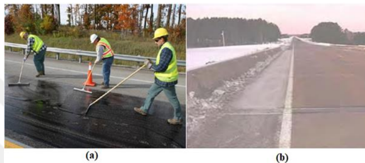
Figure 1.3 (a) The application of PC with epoxy as a cover, and (b) The difference between repaired and unrepaired pavements [9]
